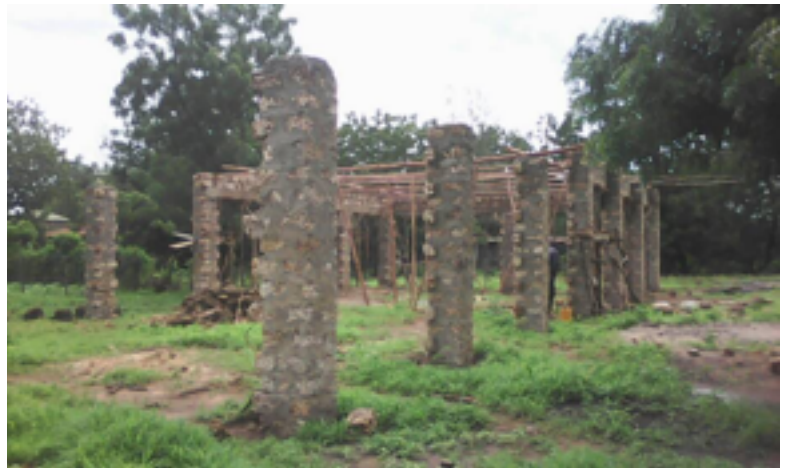
New Mpeketoni Church Needing Roof $3000
